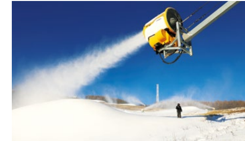
Snow-making equipment in the National Alpine Skiing Centre
