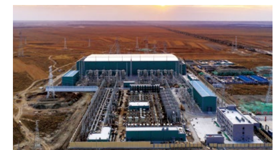
Zhangbei Converter Station
