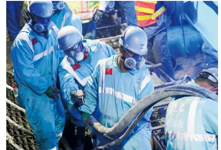
On 27 October 2018, Xiang Maosheng, the captain of the shotcrete crew of the sliding track at the Yanqing National Sliding Centre, was spraying shotcrete with a spraying gun. (Photo by the Media and Communications Department of Beijing 2022)
